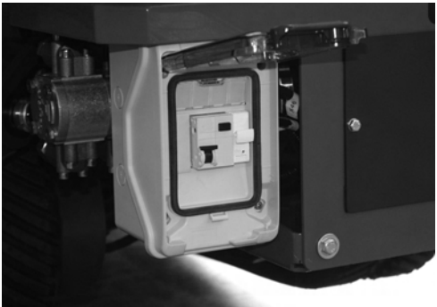
Fig. 81 Main electric switch
