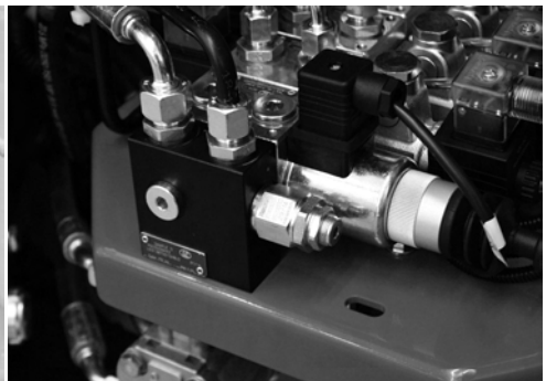
Fig. 9 Ground part pressure relief valve 1
