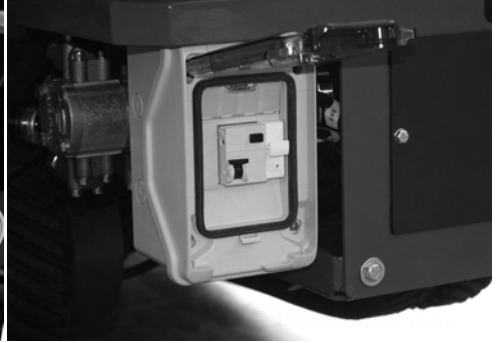
Fig. 146 Main supply switch
