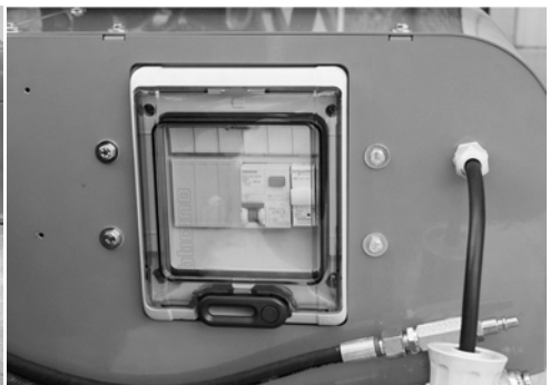
Fig. 87 Main electric switch
