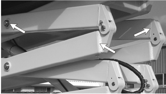
Figure 7.19 - Structural Damage and Welds
