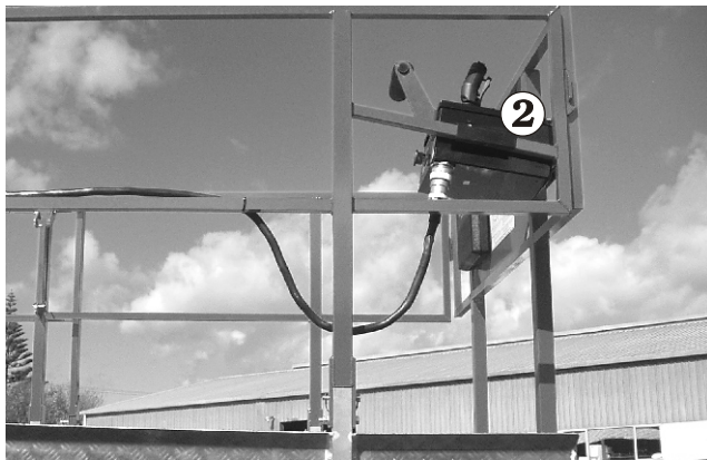
Figure 6.1.2 - Control Box Location, Platform Position
